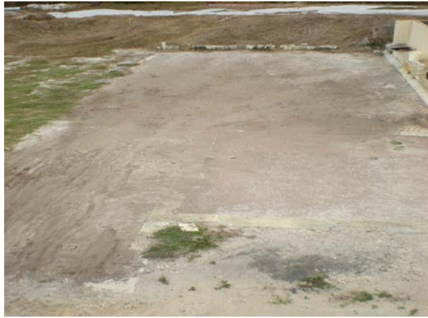
Figure 16: Pavements post loading of sandy soil
